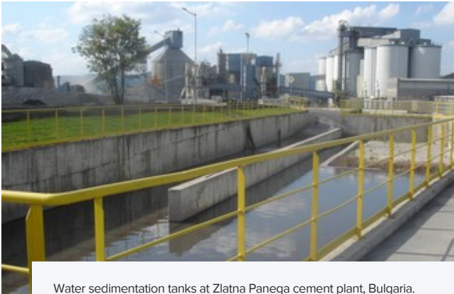
Water sedimentation tanks at Zlatna Panega cement plant, Bulgaria.
