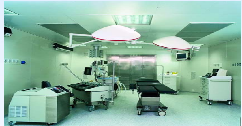
Operating Theatre at "Kyanous Stavros" General Hospital in Thessaloniki
